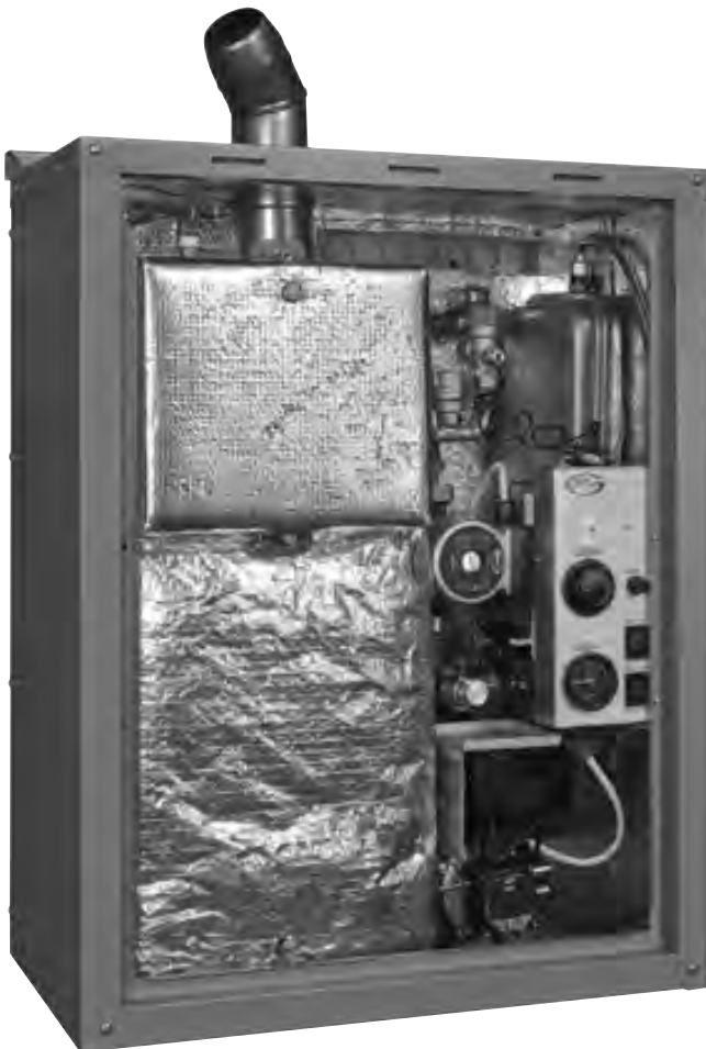
Figure 1-1: Boiler with front panel removed
